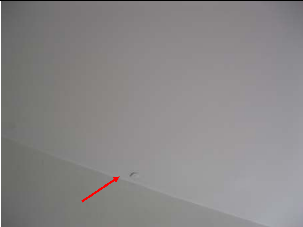
I ST251W0 Street Town Client Image # 19 Ceiling on the second floor is new sheet rock but the walls are plaster on wood lath.
