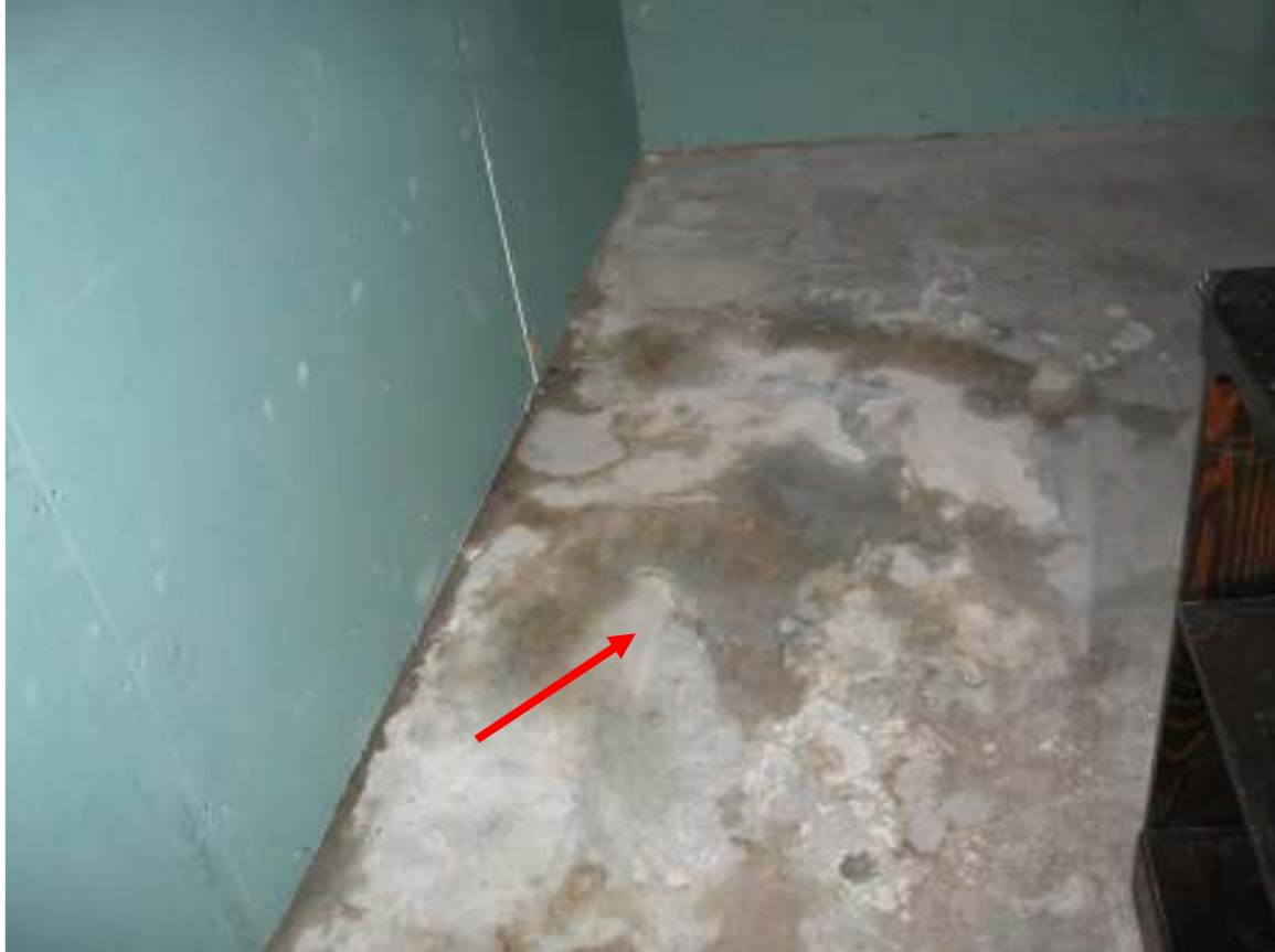
I ST251W0 Street Town Client Image# 09 Water stains on floor previous flooding
