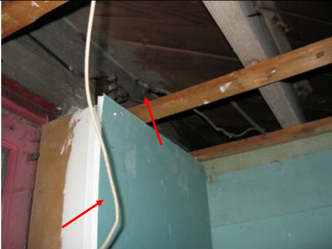
I ST251W0 Street Town Client Image # 07 Open electrical wire. Paper base sheetrock glued to the basement walls. Loose electric wiring
