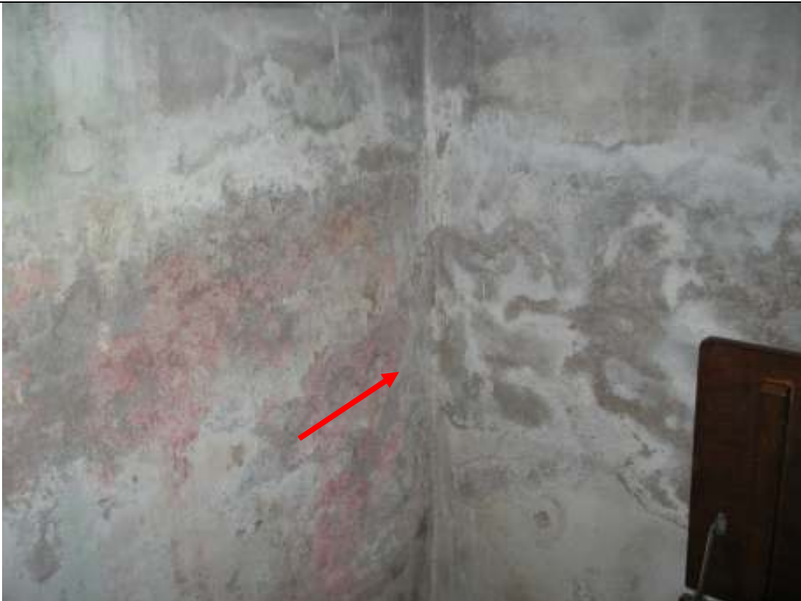
I ST251W0 Street Town Client Image # 14 Water penetration the basement walls
