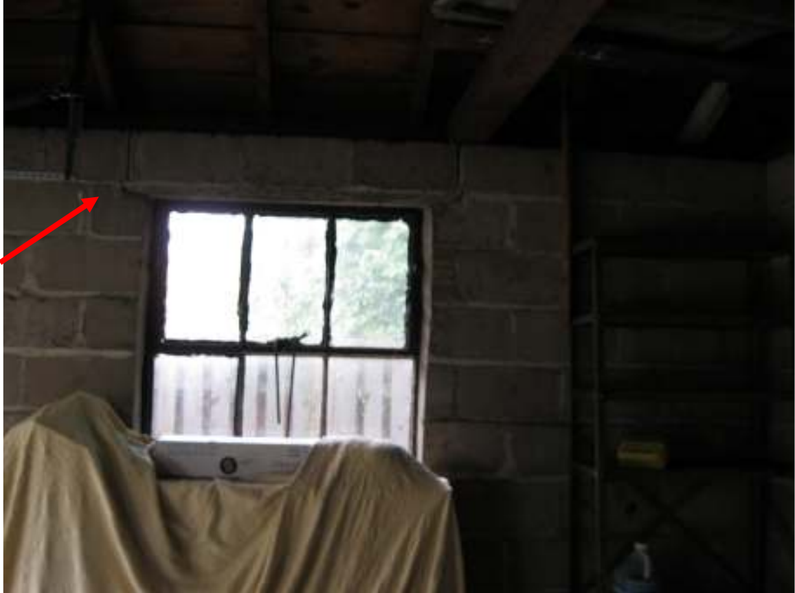
I ST251W0 Street Town Client Image # 23 Cracked bock wall above window in garage
