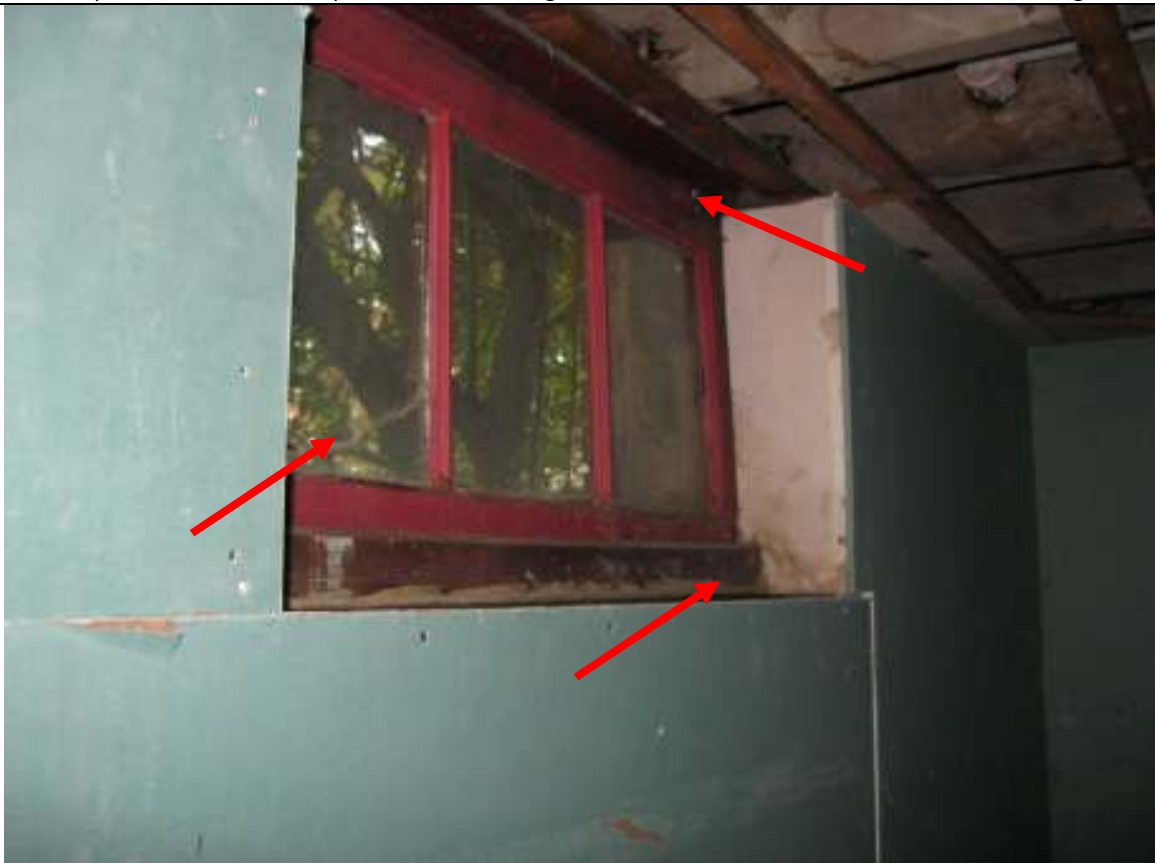
I ST251W0 Street Town Client Image # 08 Broken basement window glass. Leaking at the sill
