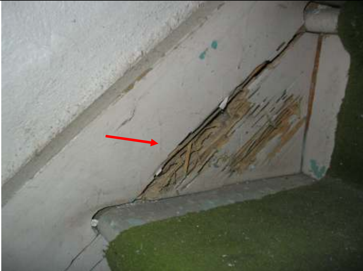
I ST251W0 Street Town Client Image # 05 Staircase stringer is termite infested
