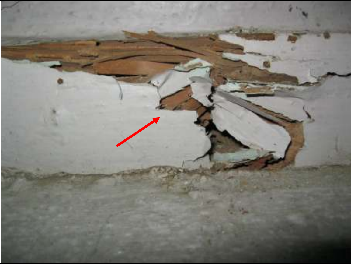
I ST251W0 Street Town Client Image # 13 Termite infested sill plate
