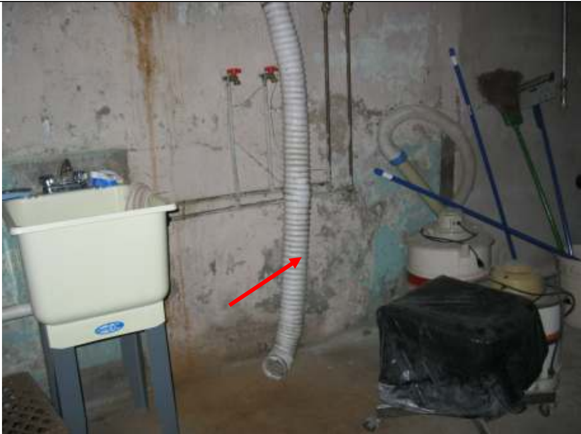
I Image Street Town Client # 10 Water penetration into basement. No laundry appliances
