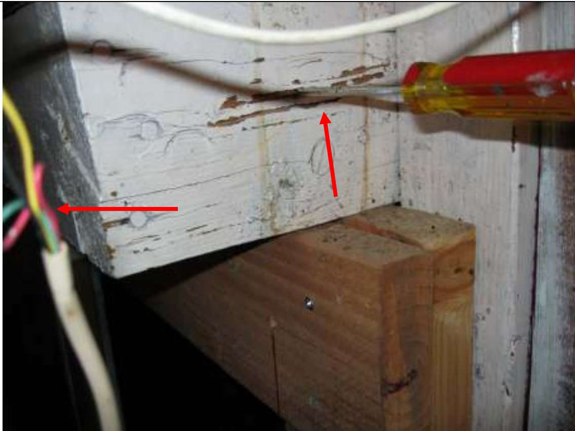
I ST251W0 Street Town Client Image # 04 Staircase to the basement is termite infested. Entire screw drive shaft penetrated. Loose Electrical wires etc
