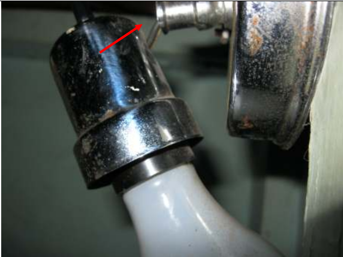
I ST251W0 Street Town Client Image # 06 Electrical lamp is broken at base. No lens
