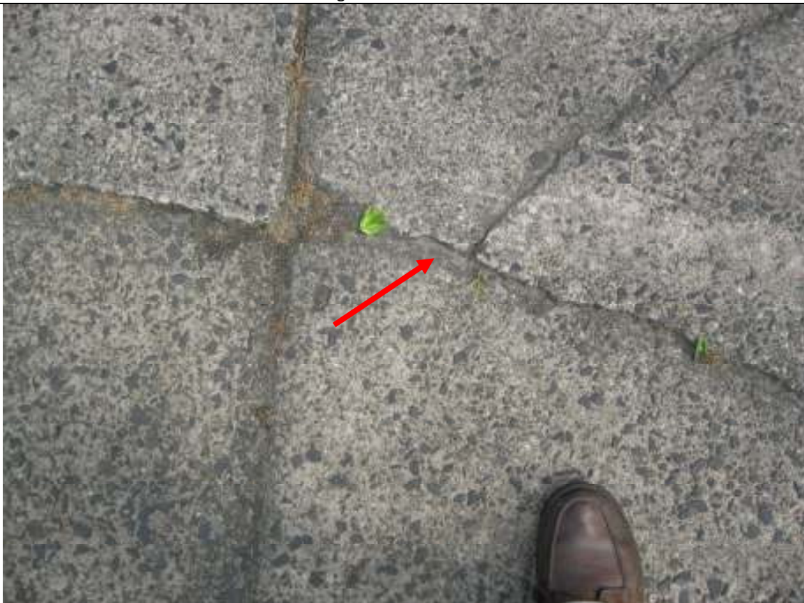
I ST251W0 Street Town Client Image # 22 Asphalt and concrete driveway is cracked
