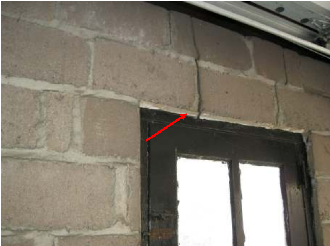
I ST251W0 Street Town Client Image # 24 Cracked concrete block wall above the door
