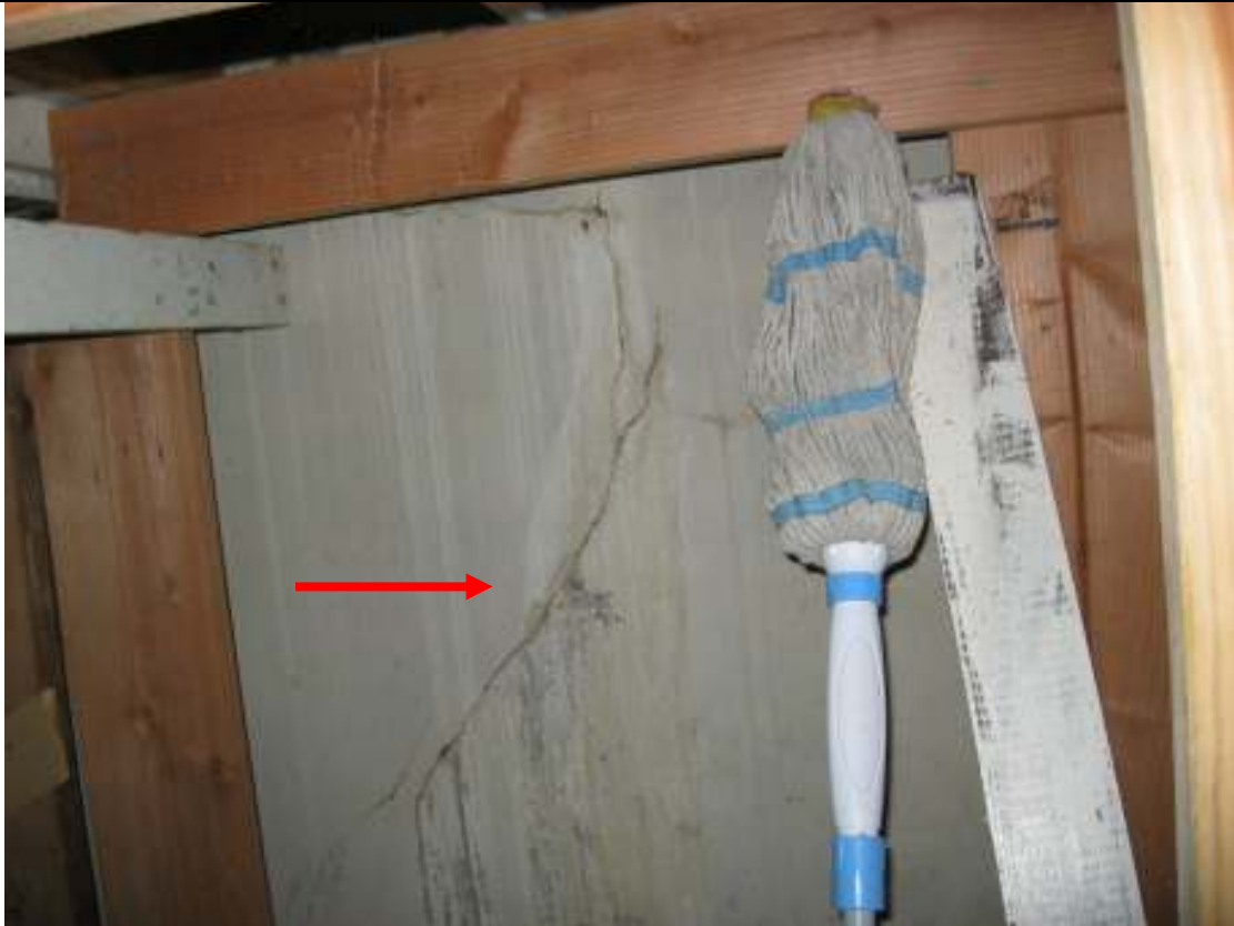
I ST251W0 Street Town Client Image # 03 Crack in the basement wall (left side)
