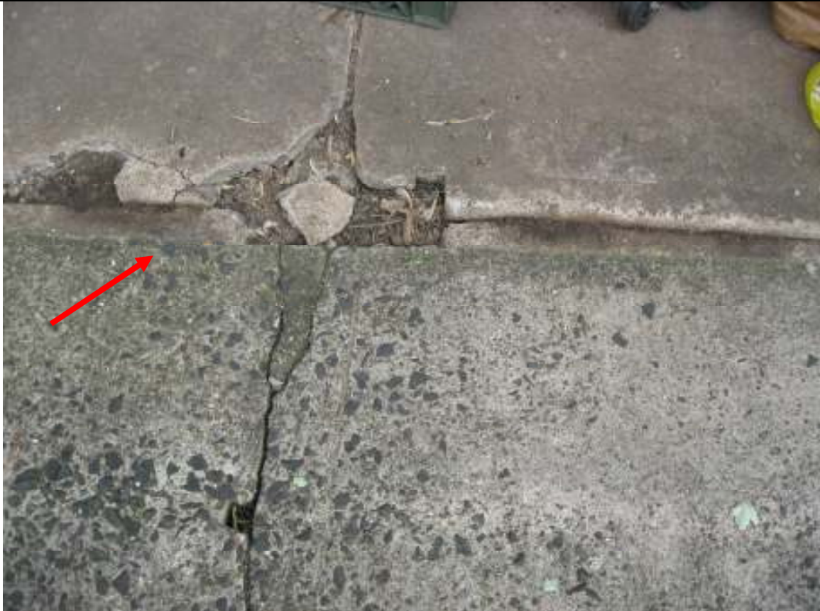
I ST251W0 Street Town Client Image # 21 Garage floor slab is cracked
