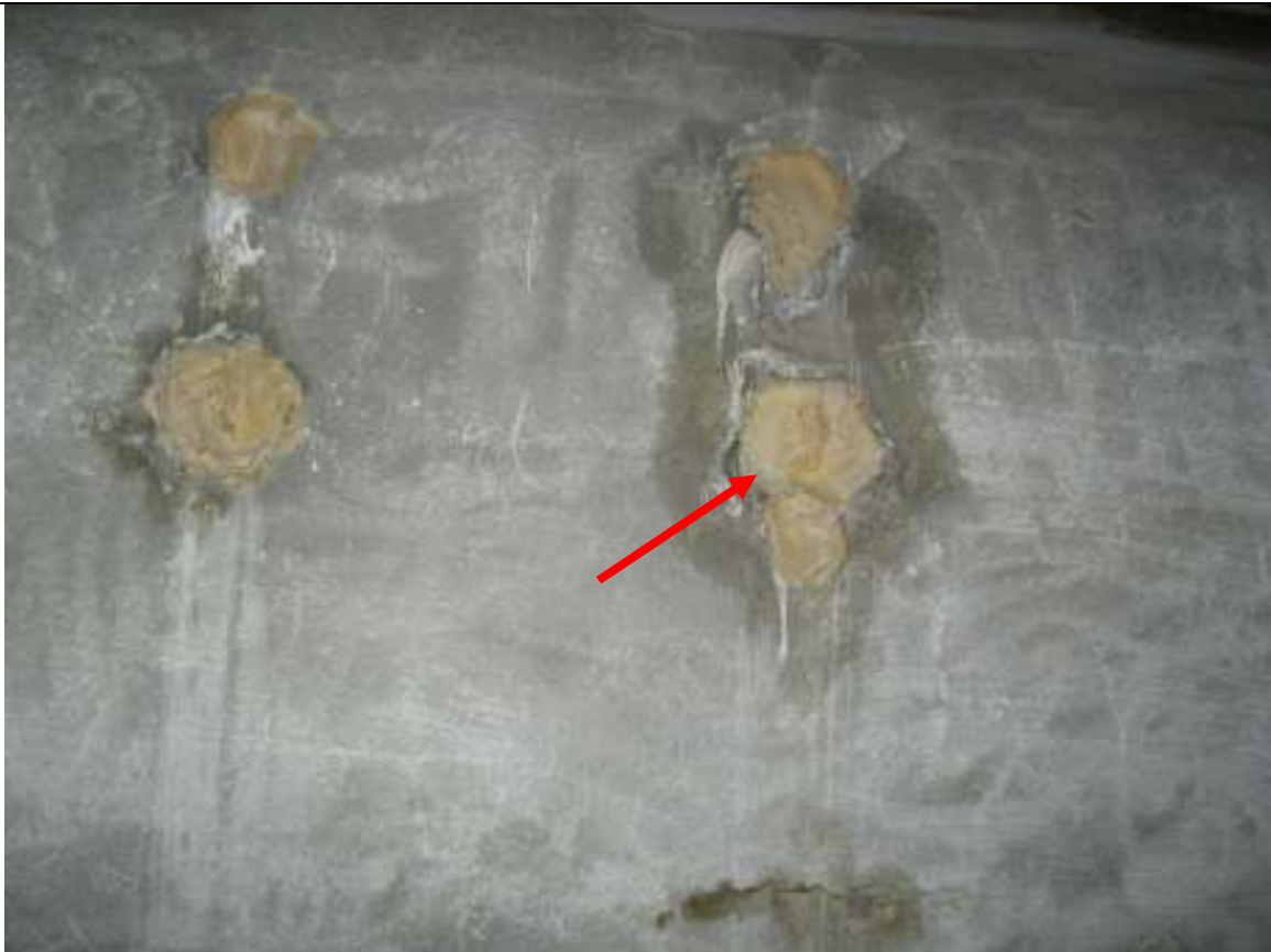
I ST251W0 Street Town Client Image # 16 Previous oil tank lines penetration through these lines
