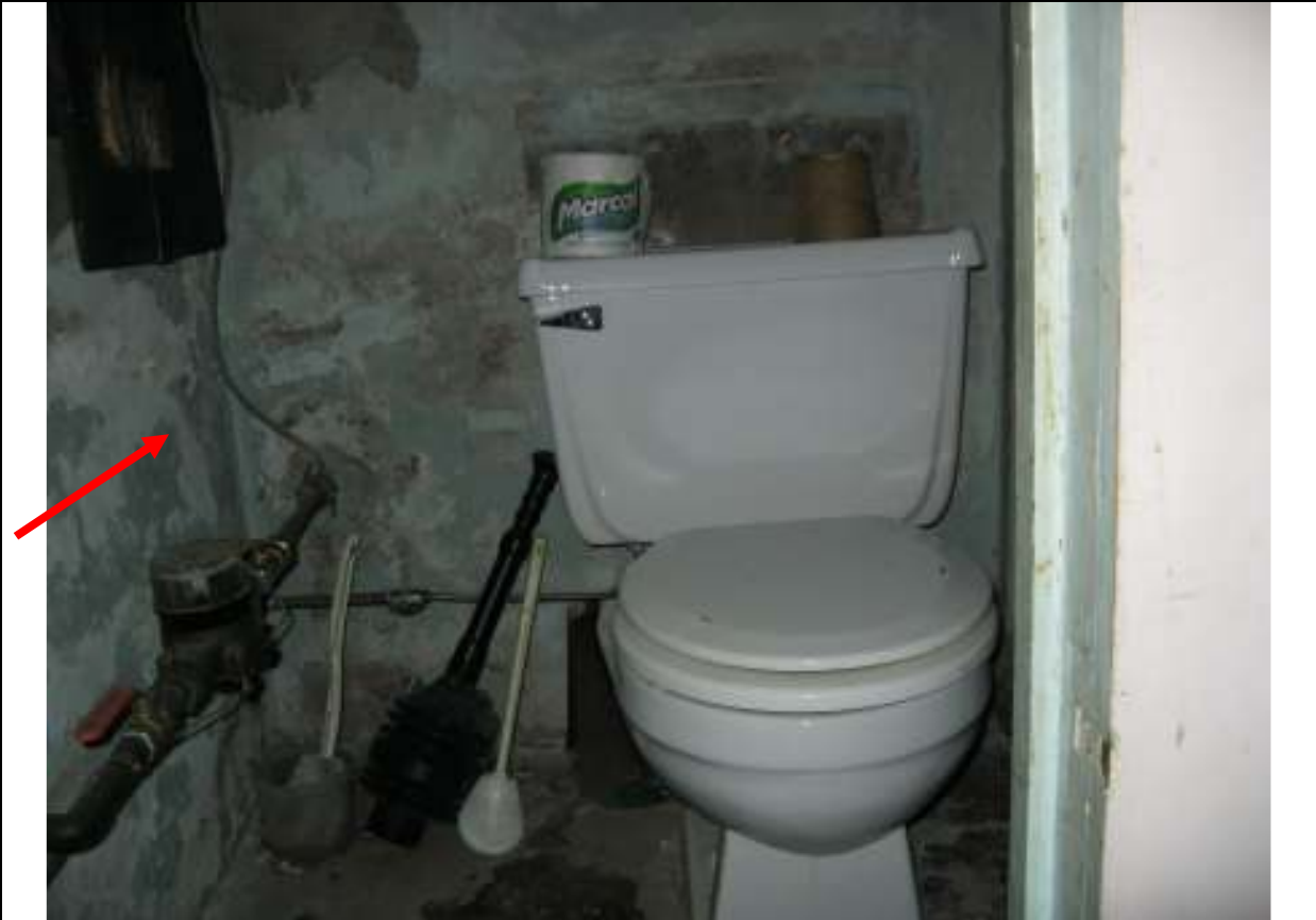
I ST251W0 Street Town Client Image# 11 Water penetration in basement. Water closet raised 12"+ above basement floor
