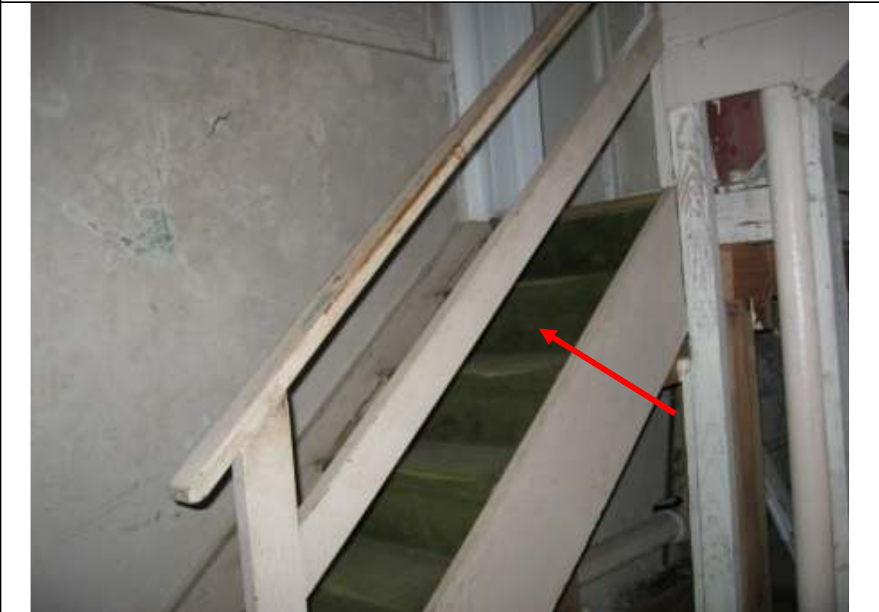
I ST251W0 Street Town Client Image # 12 Staircase railings do no meet current construction standards
