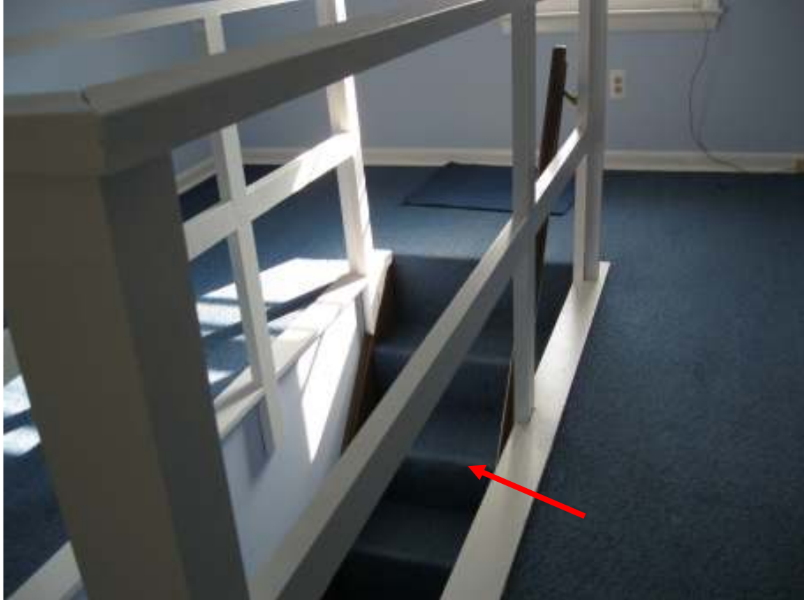
I ST251W0 Street Town Client Image # 17 Stair case guard railings in the attic do not meet current construction standards
