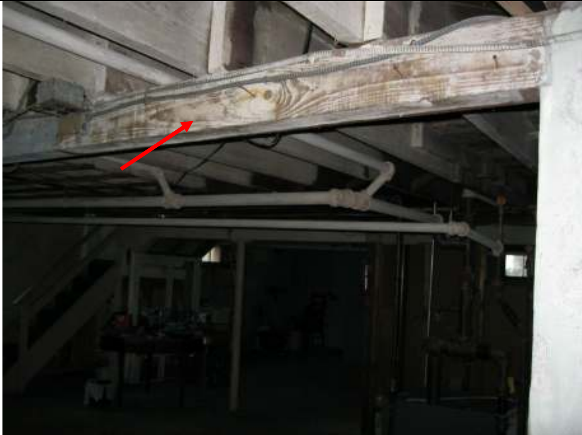
I ST251W0 Street Town Client Image # 15 Joists have been primed after the fire damage. Undersized beam (load bearing wall has been removed)
