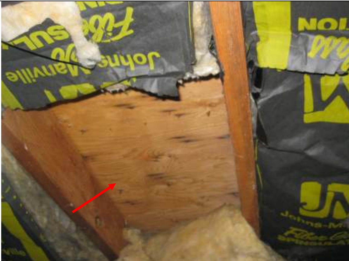
I ST251W0 Street Town Client Image # 18 Roof decking has been replaced with plywood after the fire in the top level. Insufficient Insulation
